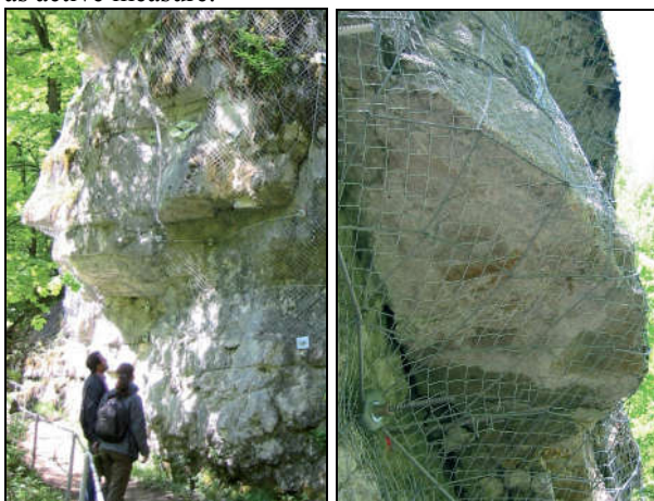
Fig. 12 – Taubenloch Canyon near Biel, Switzerland, rock protection of overhang above a hiking trail with secondary mesh
